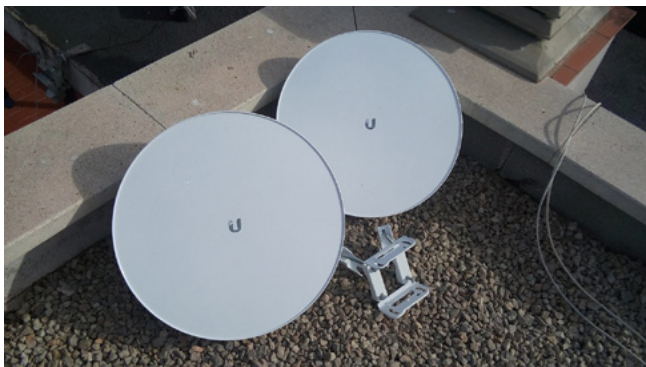
Installation of a “supernode” of Guifi.net’s network in the neighbourhood of Sant Pere i Sant Pau in Tarragona. This image by Lluís tgn is licensed under CC BY-SA 4.0
